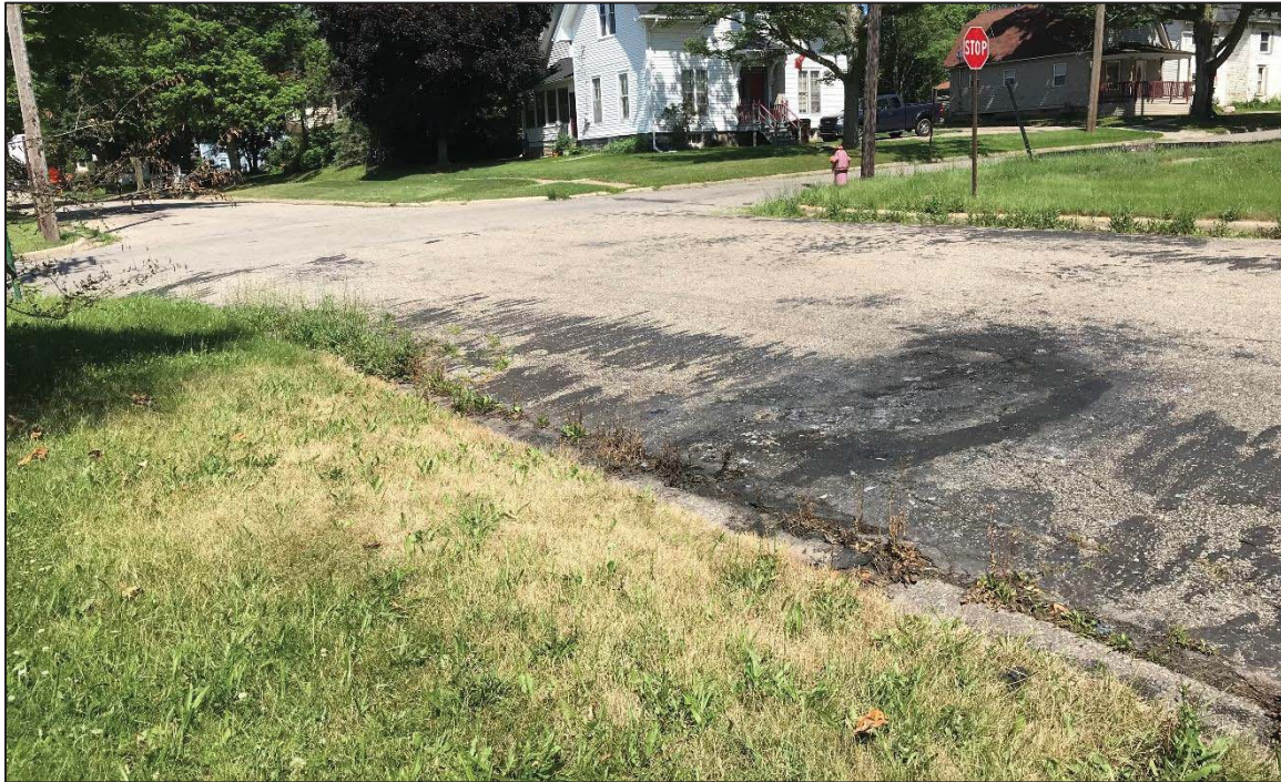
PHOTO NO. 5: View of apparent fire-damaged asphalt on East Chestnut Street and stressed grass located near the northwestern corner of the Property.
