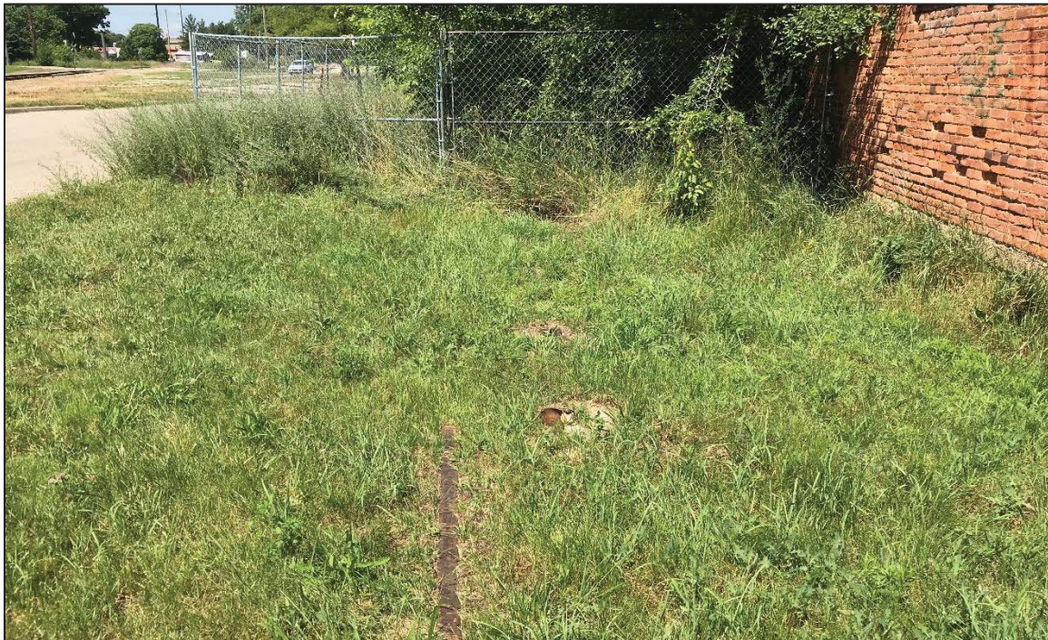
PHOTO NO. 14: View of two damaged monitoring wells observed on the southeastern corner of the Property.
