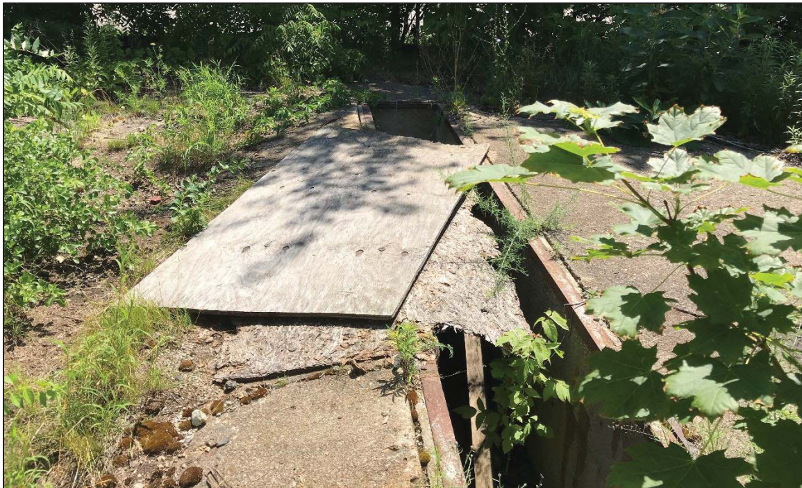
PHOTO NO. 12: View of the trench observed in the eastern portion of the Property.
