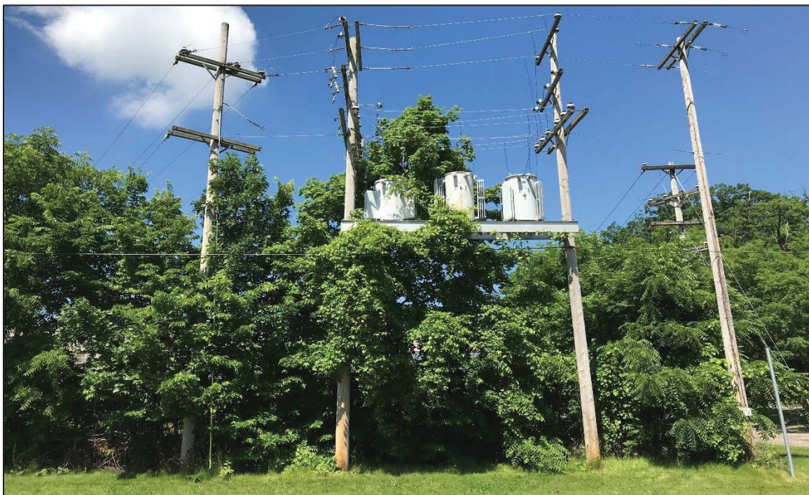
PHOTO NO. 8: View of three elevated platform-mounted transformers located on the northeastern corner of the Property.
