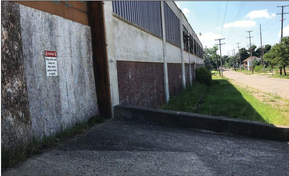
PHOTO NO. 3: View of the western side of the building on the Property, looking south.
